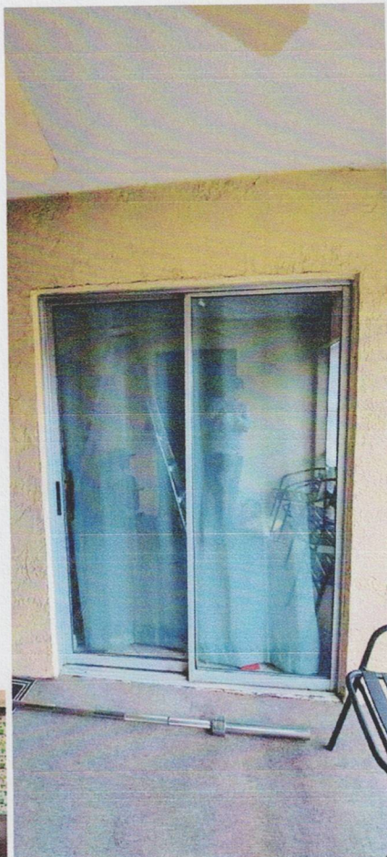
Unprotected glazed entry door
